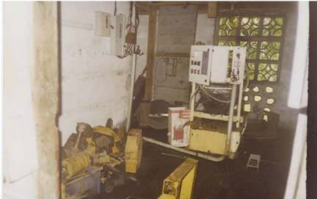
Before: what was left after the previous equipment was looted
